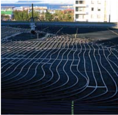
Pipe system for snow melting
