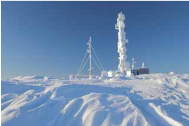
Cellular phone station.
